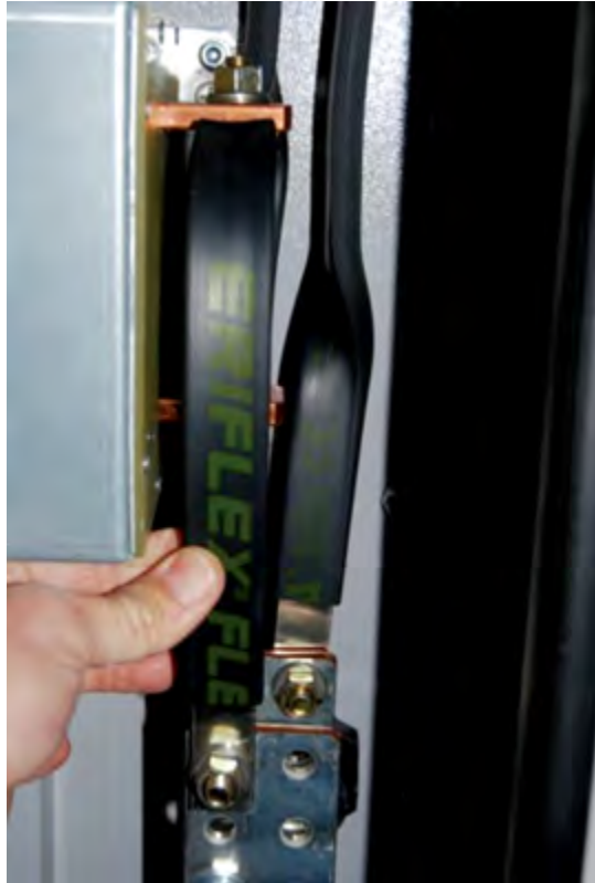
Figure 4-1. Inspection of the bus bar connection
